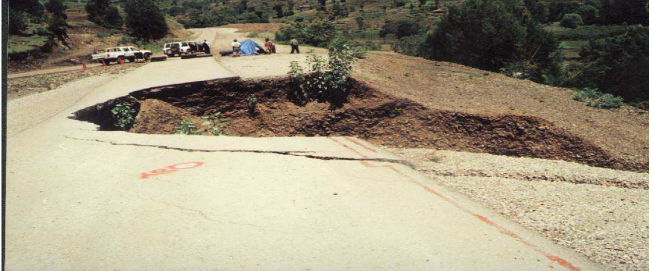
Fig. 3.2. Land slide along Bordede-Harar Road project
