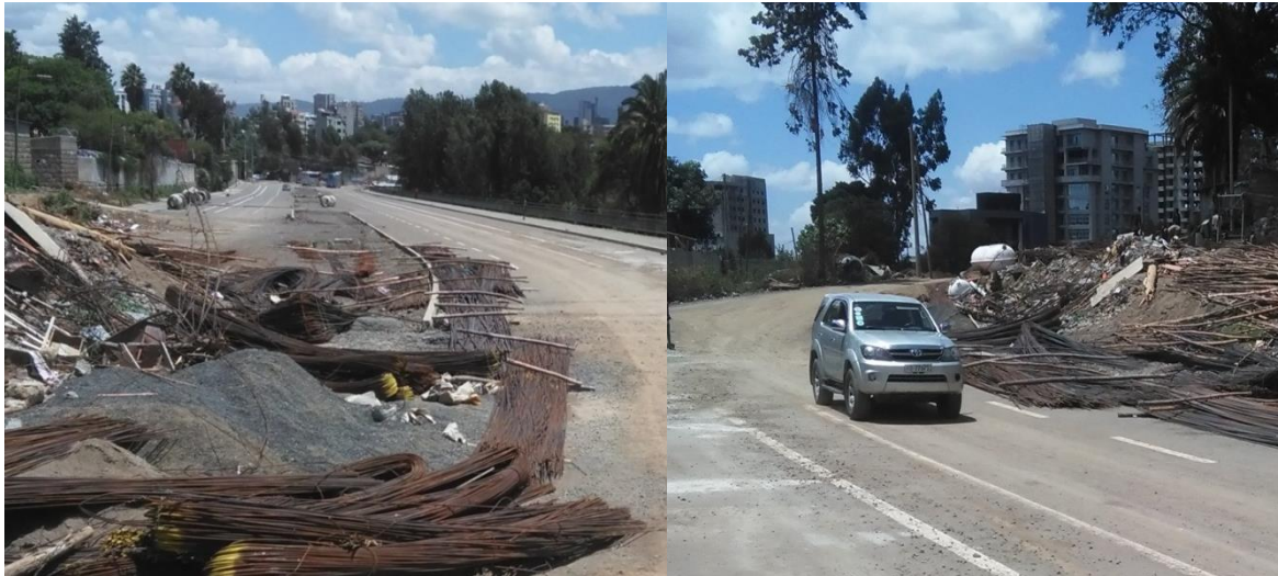
Photo 4: The road construction stops and building site holds bulk materials storage for near side construction site
