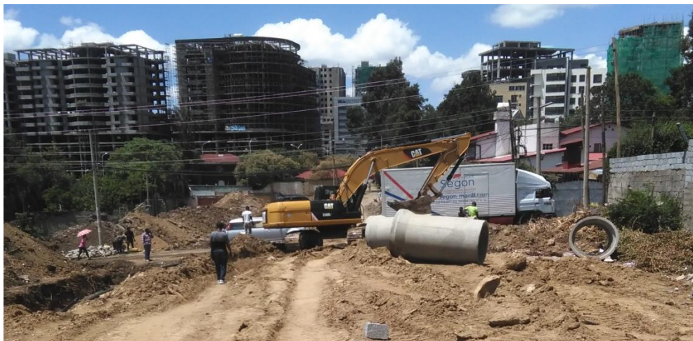
Photo 6: The road construction on progress but property not yet acquired by the agency
