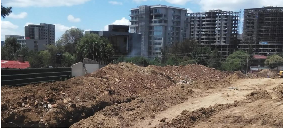
Photo 5: The road construction stops and backfill lay over the top of borrow, and low access to move construction material from one position to the other and delay happen due to delay in Row acquisition
